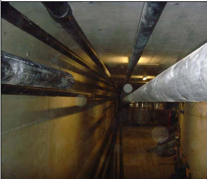
External PT Cables 27-06 BBR CME
